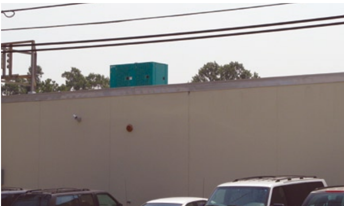
Rooftop installations, when possible, represent one solution to elevating a standby generator above flood waters in low-lying areas.
