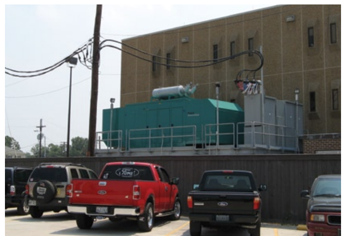
This platform installation takes advantage of a unique space created by a retaining wall in an urban area.
