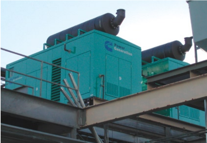
These generators are located on a high superstructure in an area where flooding is likely during severe weather.
