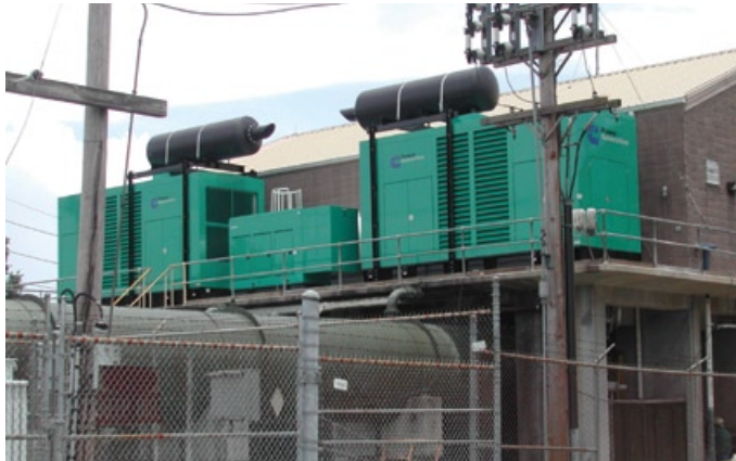
Three Cummins Power Generation generators at a Jefferson Parish canal pumping station were located above the maximum high-water level and continued to operate as long as they had fuel.
